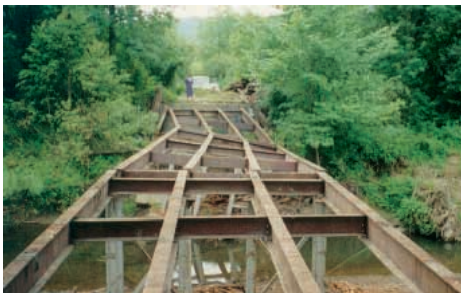
Fot. 1. Widok na zniszczony most Photo 1. View of the destroyed bridge
