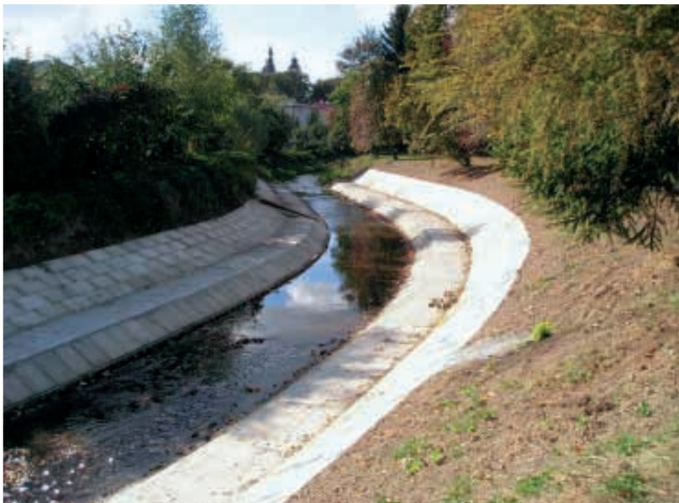
Fot. 34. Widok na uregulowania brzegowe rzeki Opatówki Photo 34. View of the Opatówka river bank regulating structures
