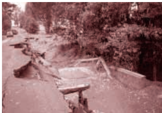
Fot. 40. Widok na oberwane pobocza drogi Photo 40. View of the destroyed road shoulders
